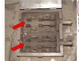
Figure L Black panel 2no. Internals To knife switch box - wooden boxing Chrysotile
