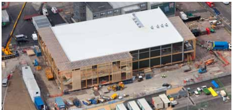
Aerial view of the Olympic Park showing the construction of the new McDonald's restaurant, April 2012
