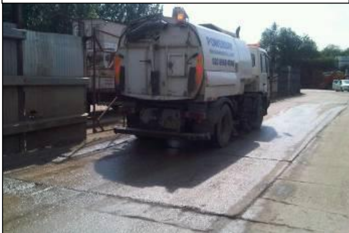
Figure 6.3: Neasden Lane Industrial Site: Internal haul road with privately run sweeper, which also applied CMA
