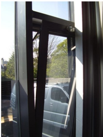
Figure 5.2 Example of ventilation area reduced by the restrictor. Column prevents window opening
